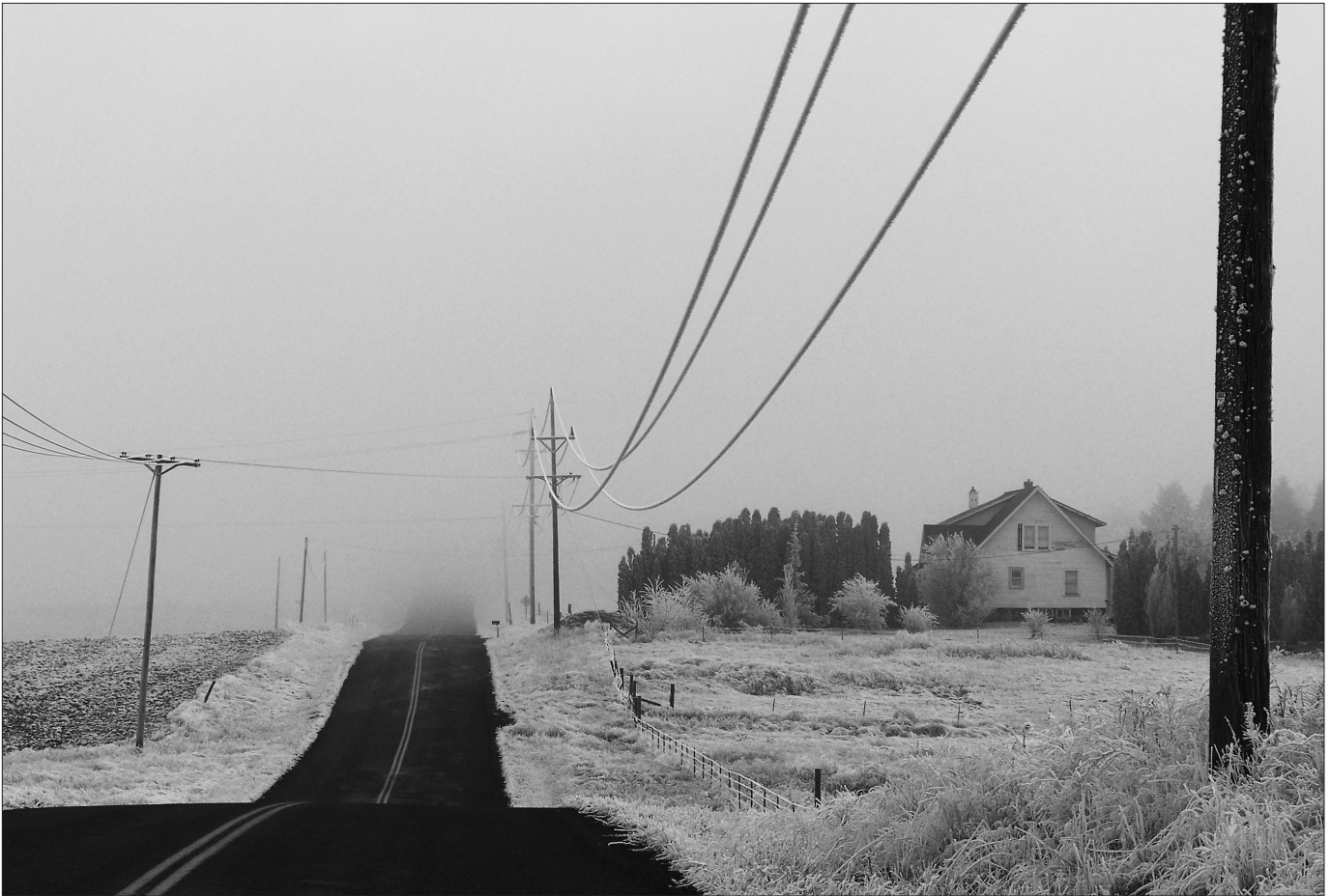
Above, power lines in Klickitat County sag from the weight of a December frost. Below, line Foreman John Starr, left, and Lineman Todd Niva retie wire on a crossarm.
